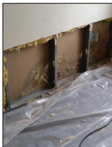
Photo courtesy of Linda Mozden Facilities has had to remove walls to stop mold from continuing to grow.
