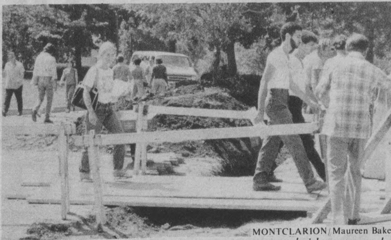
DETOUR! students must now use a temporary bridge to pass by construction that is underway on underground steam pipes near the library.
