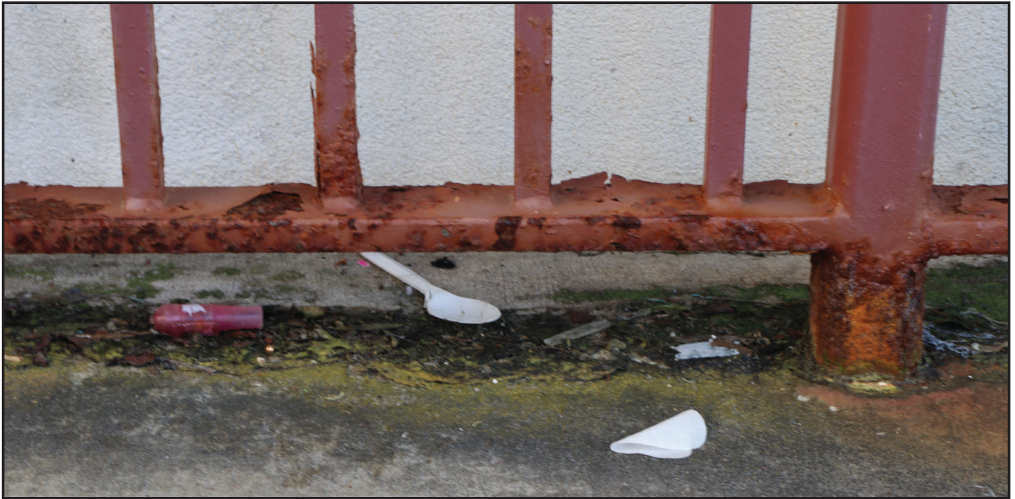
A rusty rail on the steps leading up to the entrance of Machuga Heights.
